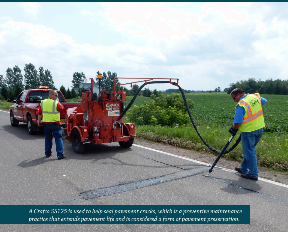
An Etnyre distributor mounted on a Peterbilt truck applies a cationic rapid-setting, polymer modified (CRS-2P) asphalt emulsion as part of a chip seal operation.
