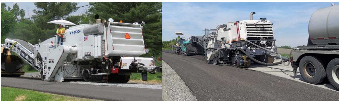
(a) (b) Figure 12 Single unit CIR Trains (courtesy ARRA)
