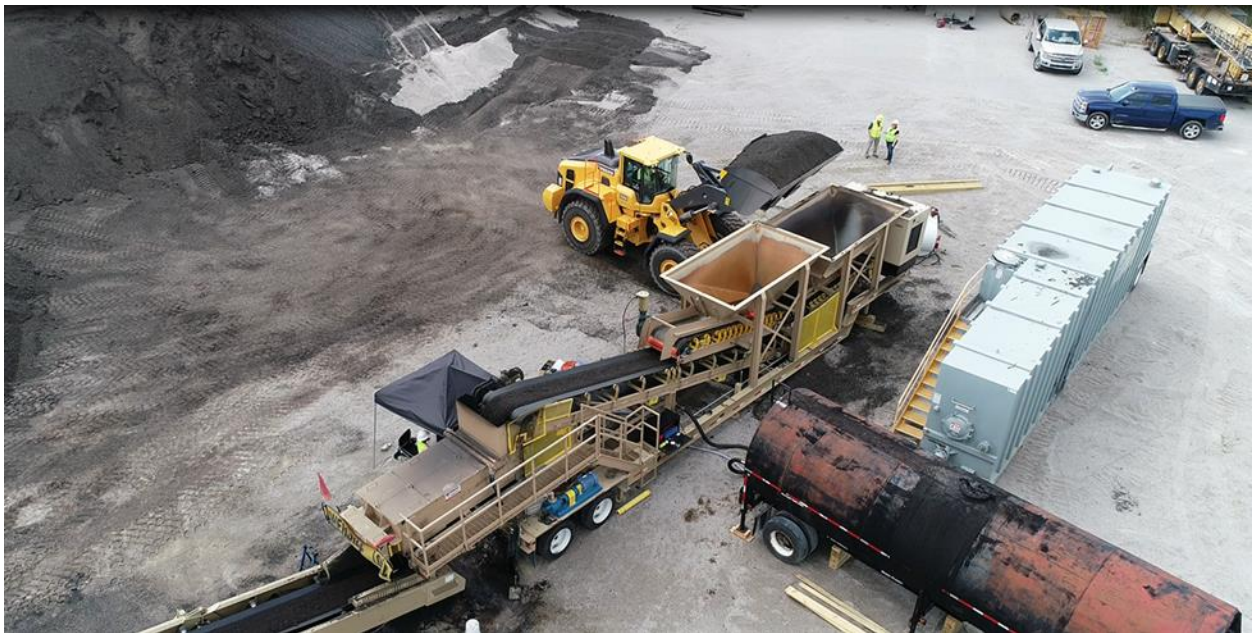
Figure 18 CCPR Plant (Courtesy HRG)
