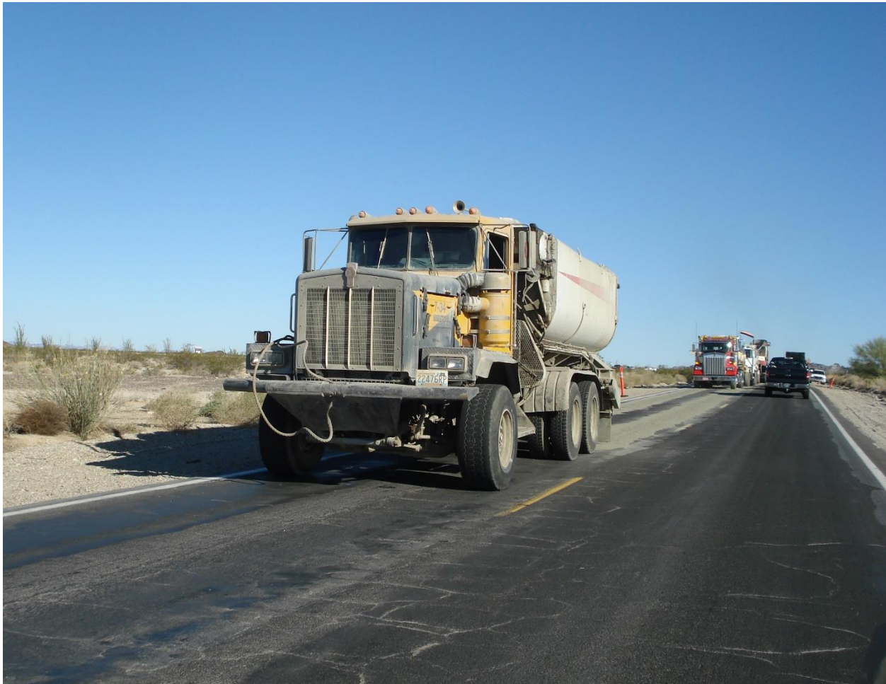
Figure 11 Applying active filler (cement) ahead of a multi-unit CIR train. (courtesy ARRA)
