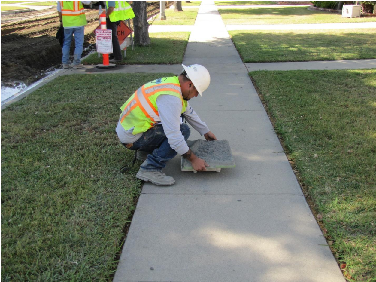
Figure 22 Measuring the application rate of active filler using a pan test. (courtesy ARRA)
